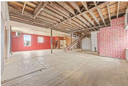
Basement featuring wood-type flooring and a wall mounted AC
