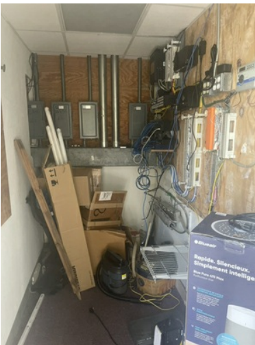
Interior View - Electrical
