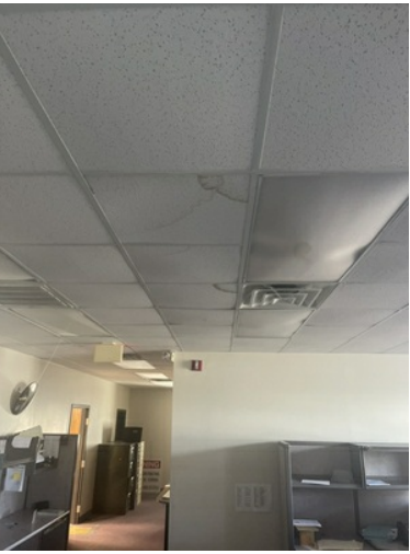
Interior View - Ceiling Damage
