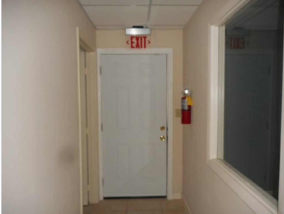
Exit Door / Extinguisher
