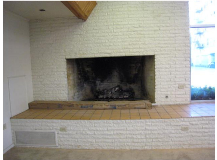
Gas Log fireplace in reception area
