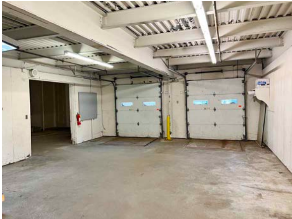
Overhead Doors in Back Storage Room
