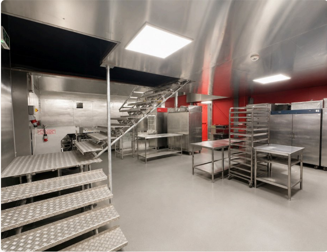
Production floor · Stainless lining, column-supported
