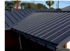
Metal Roof- Black- Standing seam
