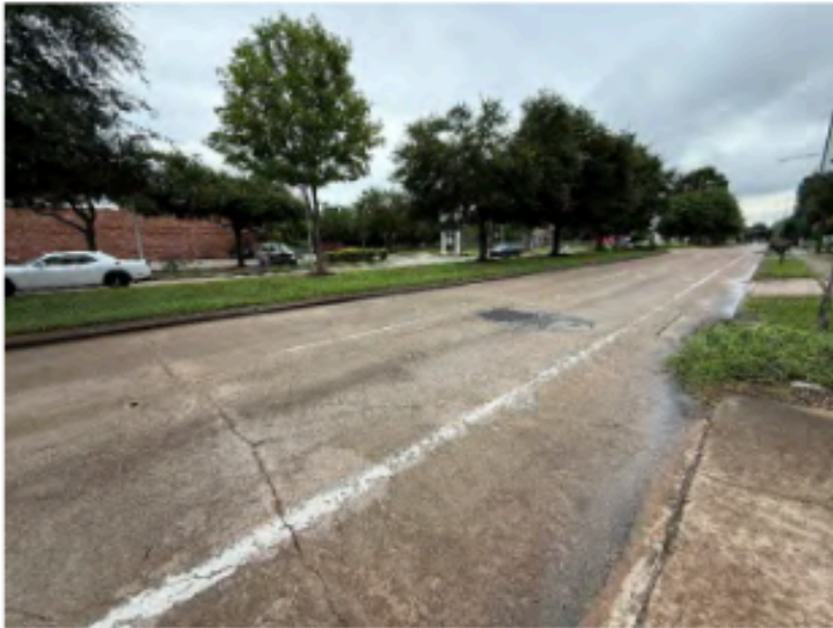
Blalock Road Looking South
