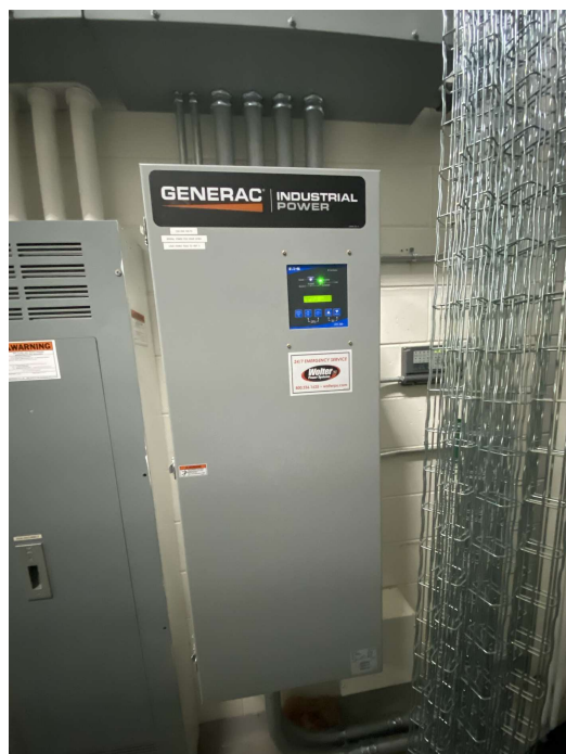
GENERAC 130 kw w/Auto Switching
