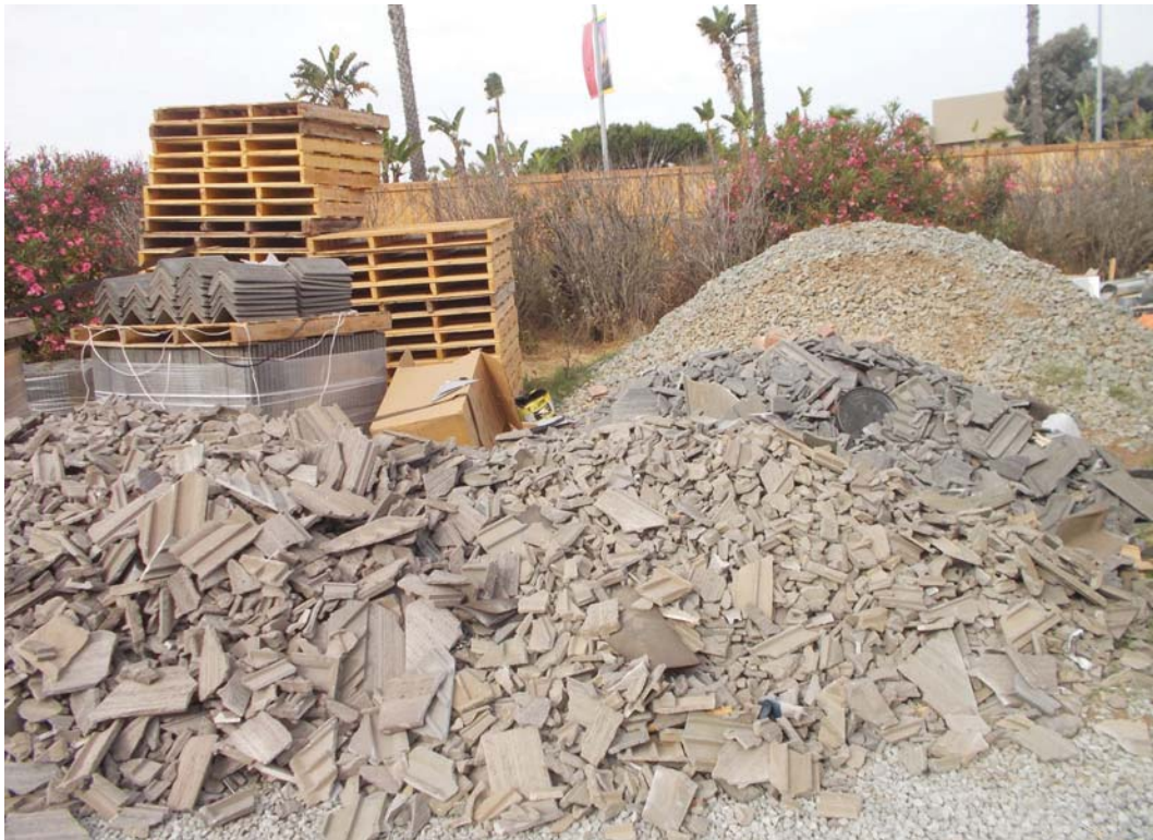
2) View of typical debris piles on vacant portion of Site.
