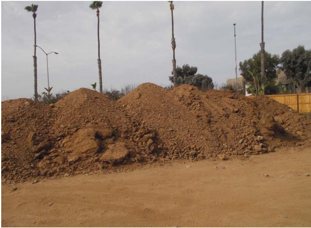
1) View of typical soil piles on vacant portion of Site.
