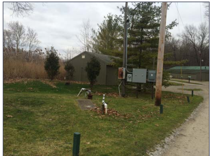
480 square foot pump house
