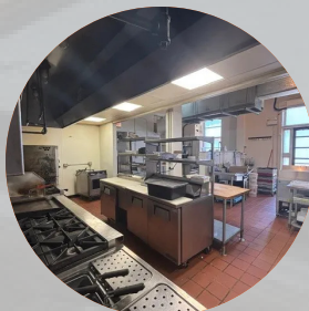
In Place Commercial Kitchen
