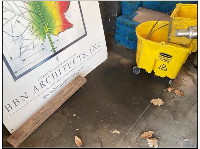
26. Interior – shop, staining
