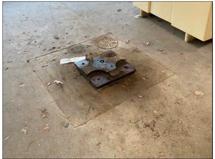
22. Interior – shop, floor drain and lift and staining
