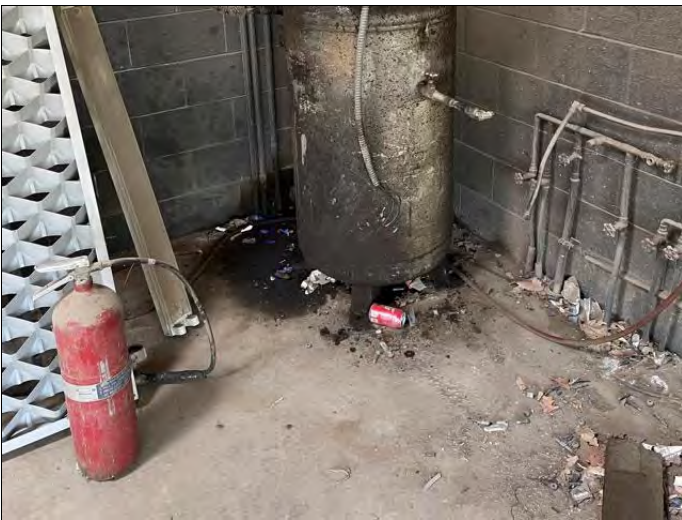
27. Interior – shop, staining
