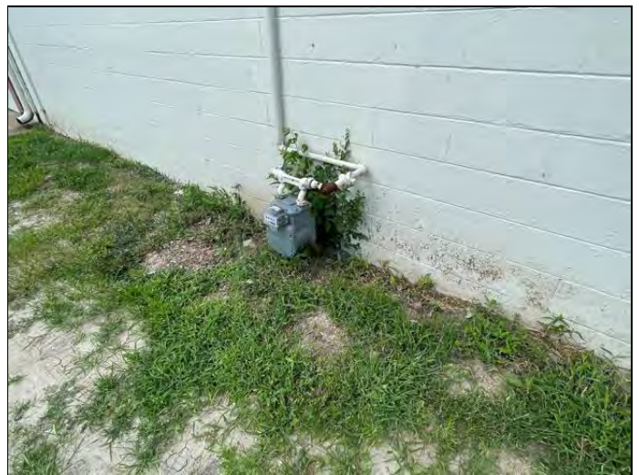
12. Natural gas connection to the Subject
