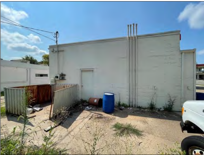
9. Oil storage drum and vent pipes
