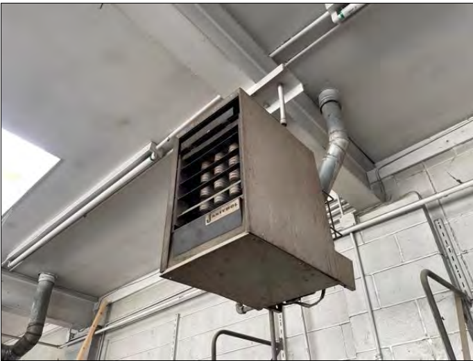
21. Interior – shop, overhead heater
