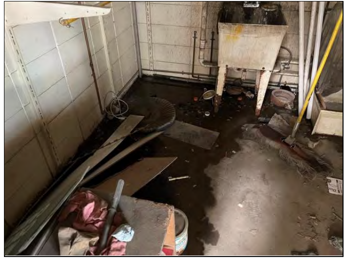
20. Interior – shop, standing water in the mechanical room
