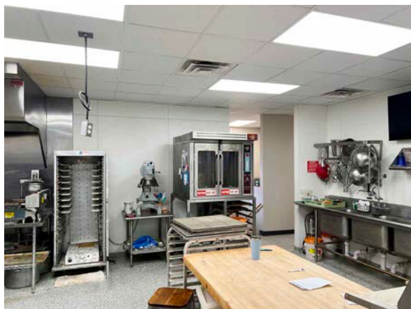
Main Level - Kitchen
