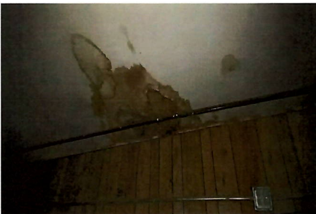
Picture 19 – Water Damage at Ceiling
