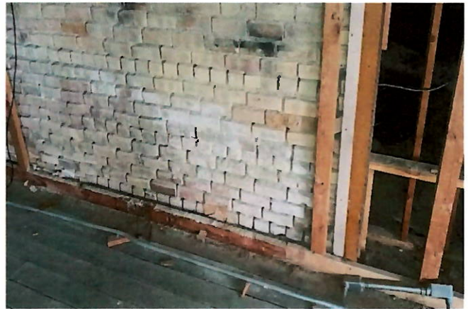
Picture 18 – Decayed Brick – First Floor
