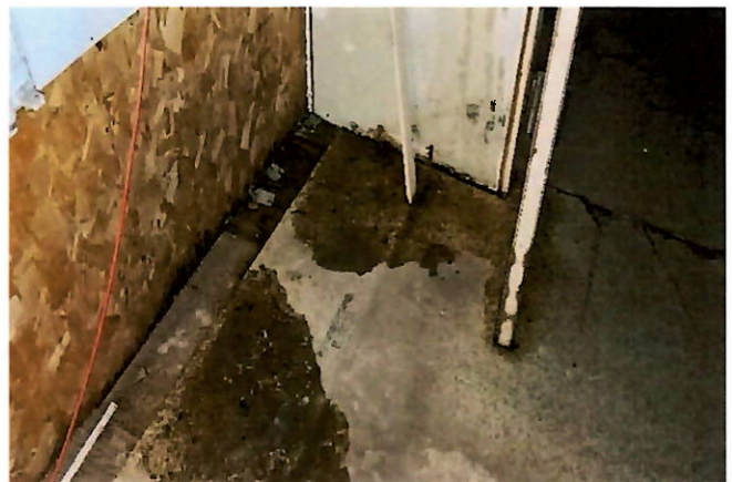
Picture 20 – Water Damage at Floor
