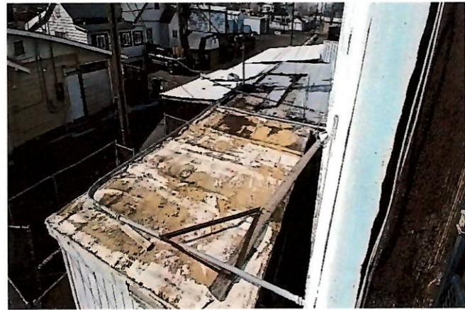
Picture 10 – Roofing Failure
