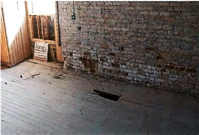
Picture 17 – Decayed Brick – First Floor
