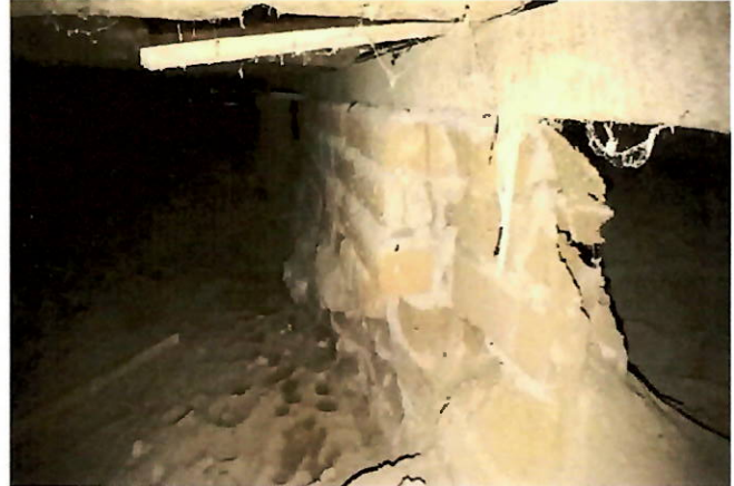
Picture 16 – Existing Floor Joists and Decayed Brick Footings
