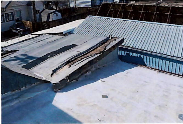
Picture 7 – Damaged Roofing
