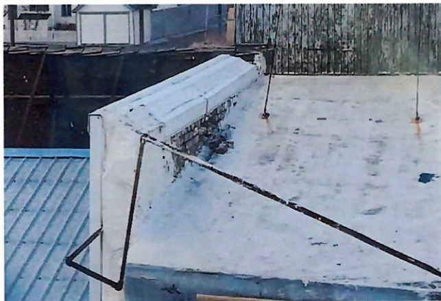
Picture 9 – Parapet Failure and Piping
