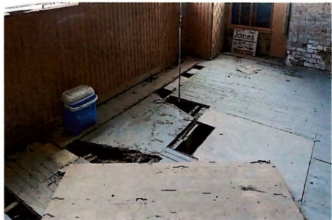
Picture 14 – Flooring Damage
