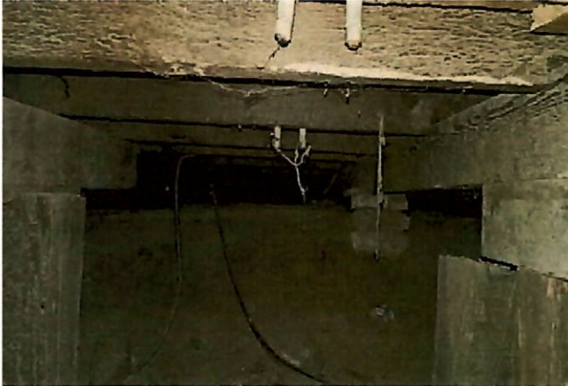
Picture 15 – Existing Floor Joists and Decayed Brick Footings
