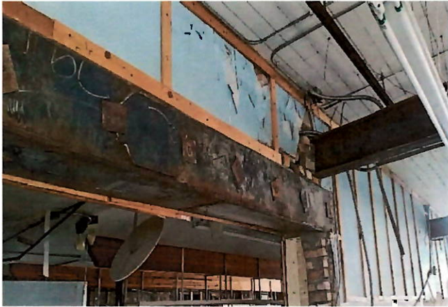
Picture 11 – Retrofitted Header
