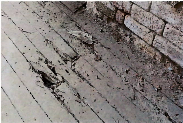
Picture 13 – Flooring Insect Damage
