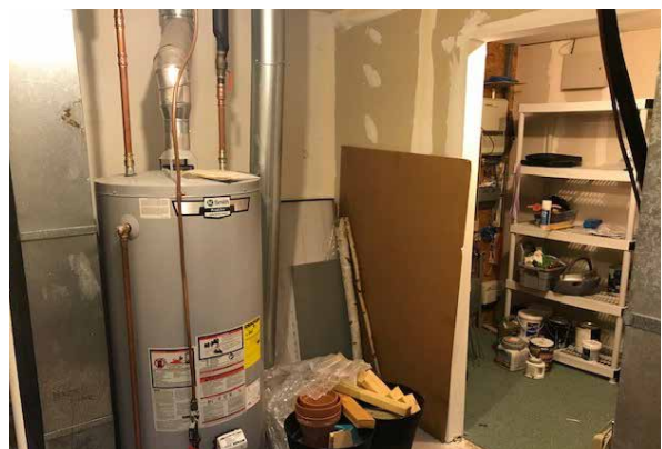
Lower Level: Shared Utility Room
