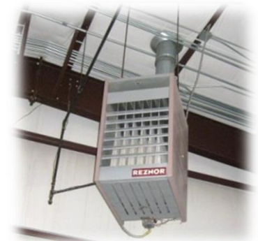
Suspended Gas Heater
