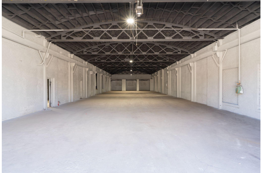
Studios will be in this room. A transom/window will be installed along the right side of the wall
