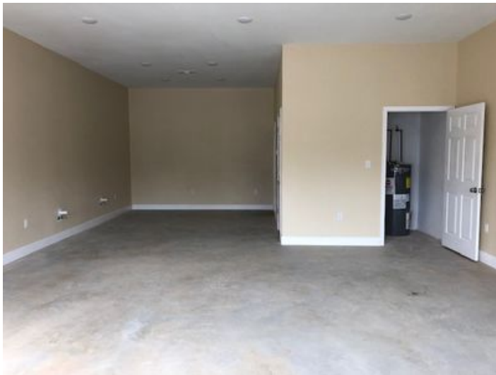
Open Gallery/Also Plumbed for Salon
