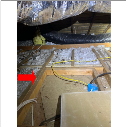
ITEM: 5:4. The attic insulation does not appear to be of adequate depth or properly installed
