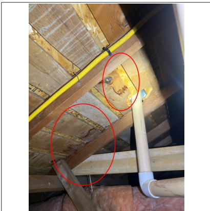
ITEM: 5:1. There are moisture stains on the roof sheathing as viewed from within the attic area
