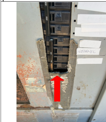
ITEM: 2:11. The dead head Cover at the main electrical service entry panel is loose and there is one or more missing circuit breaker blank cover plates
