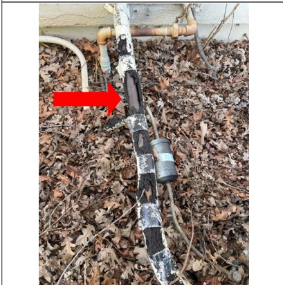
ITEM: 12:4. Sections of the insulation at the line set at both of the AC condensing units are torn and damaged
