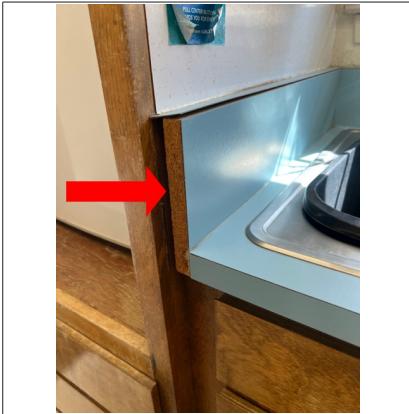
ITEM: 8:2. The edge piece at the Formica countertop in kitchen (2) is missing
