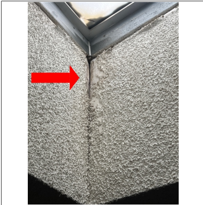
ITEM: 4:5. There is water damage visible at the back skylight area as viewed from the interior of the structure
