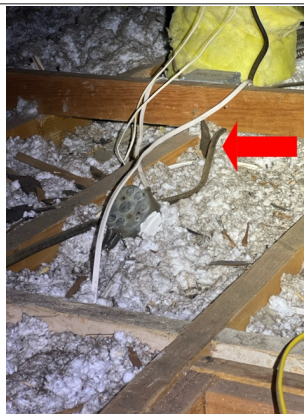
ITEM: 5:2. Portions of the wiring in the attic are loose and improperly terminated
