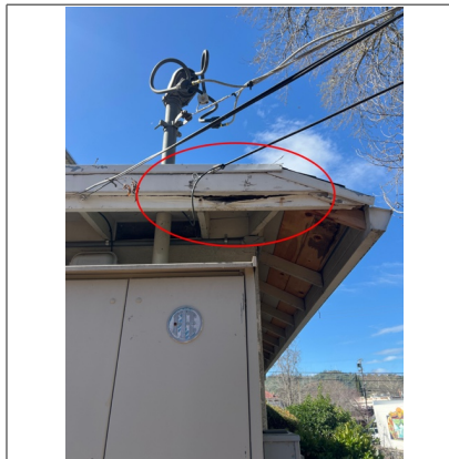
ITEM: 2:4. There is dry rot damage present at the back fascia board
