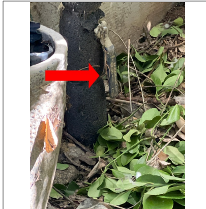
Image of the water shut off valve at the front left corner
