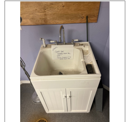
ITEM: 6:14. The sink in the basement area was not tested but appears to be loose
