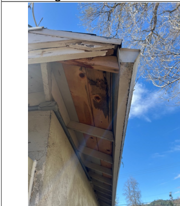
ITEM: 2:7. There are water stains noted at the wood members in the eaves which may indicate a possible roof leak
