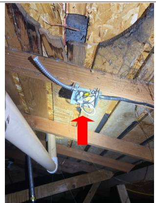
ITEM: 5:3. There are missing cover plates at one or more of the electrical junction boxes in the attic
