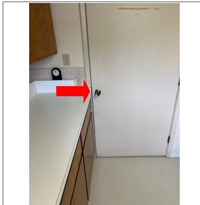
ITEM: 6:2. The entry door to exam room #1 does not properly latch
