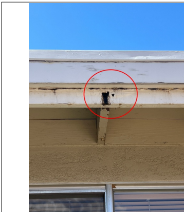
ITEM: 2:4. There is dry rot damage present at the back fascia board
