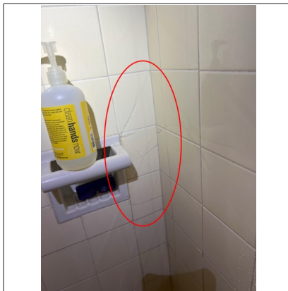
ITEM: 9:5. There are loose and cracked tiles at the private bathroom shower stall
