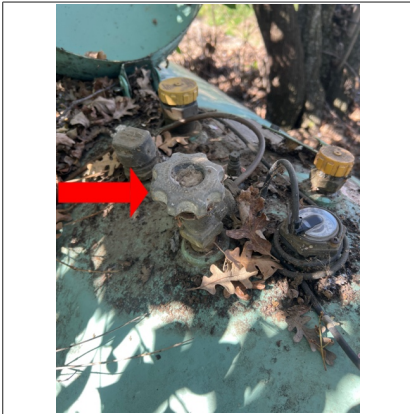
Image of the gas shut off valve on top of the tank
