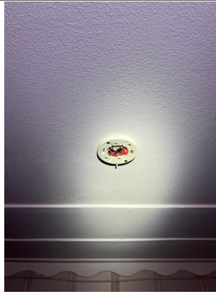
ITEM: 6:9. There is a missing cover plate with exposed electrical wires present in the ceiling of the exam room at the left center portion of the structure
