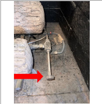
Image of the Gas shut off valve
