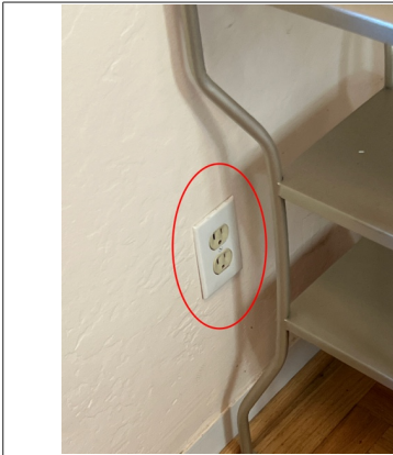
ITEM: 6:5. One or more receptacles throughout the structure have an open ground
