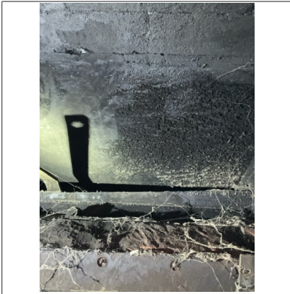
ITEM: 10:1. The interior of the fire box area of the fireplace has a build up of creosote
