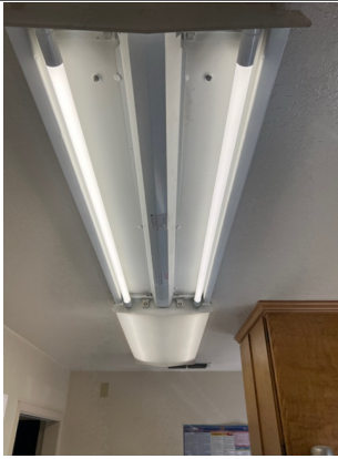
ITEM: 6:8. There are missing light lenses in one or more areas throughout the structure
