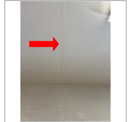
ITEM: 6:4. There are damaged and cracked sections of drywall throughout the structure
