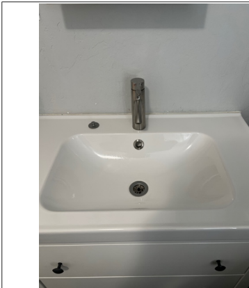
ITEM: 6:12. There is no running hot water at either of the front to left exam room sinks
