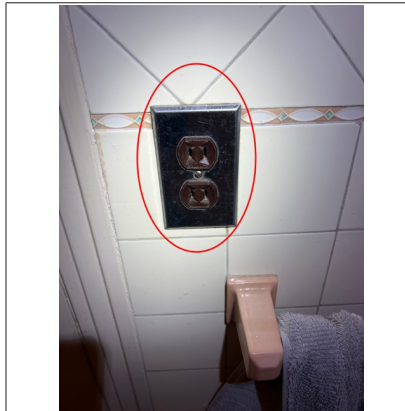
ITEM: 9:1. None of the outlets in the office and private bathrooms are GFI protected
