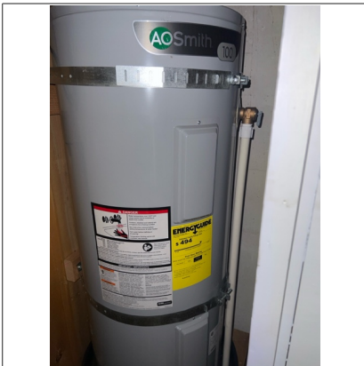
Image of the water heater
