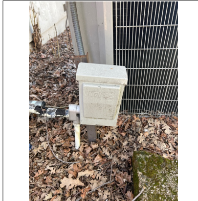
Image of the disconnect AC unit #2
