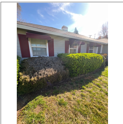
ITEM: 1:3. There are planted shrubs at the exterior which are slightly in contact with the structure
