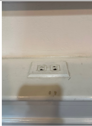
ITEM: 6:6. There are non grounded outlets installed throughout the structure
