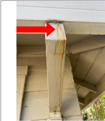
ITEM: 2:2. One or more of the gutter downspouts are stained indicating a possible leak
