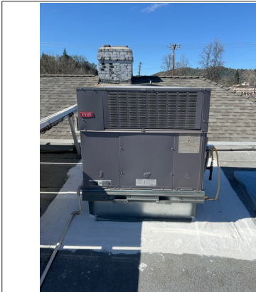
Image of the heat pump
