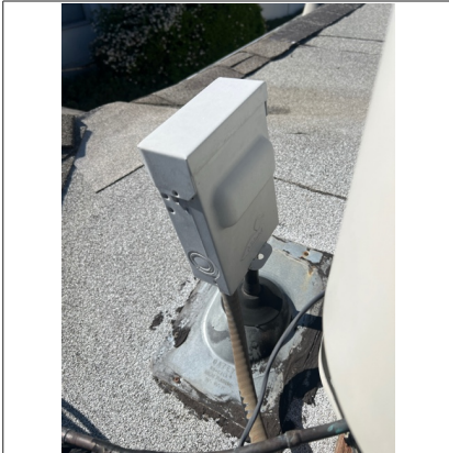
Image of the disconnect AC unit #1
