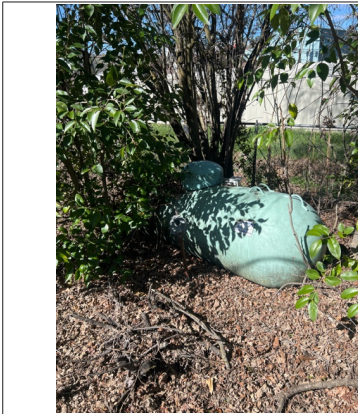
Image of the propane tank
