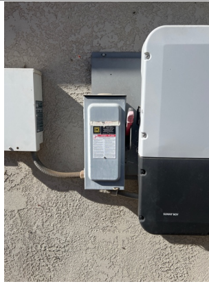
Image of the transfer switch
