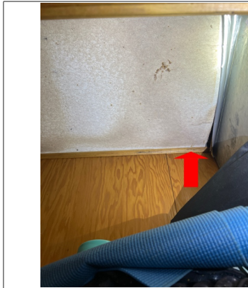
ITEM: 6:4. There are damaged and cracked sections of drywall throughout the structure
