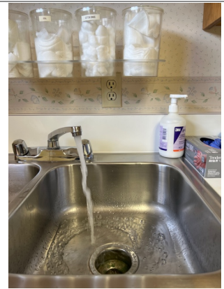
ITEM: 6:7. One or more of the outlets near the sinks in the exam rooms are not GFI protected
