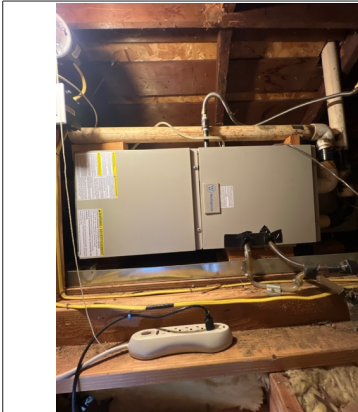
Image of furnace unit #1
