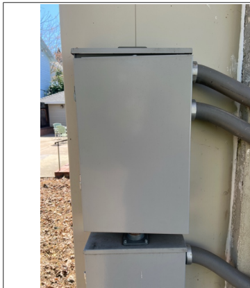
Image of electrical subpanel #1
