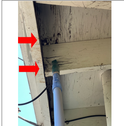
ITEM: 2:5. There is dry rot damage present at the back roof sheathing and rafter tails
