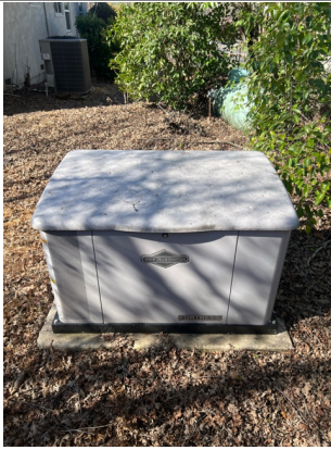
Image of the generator
