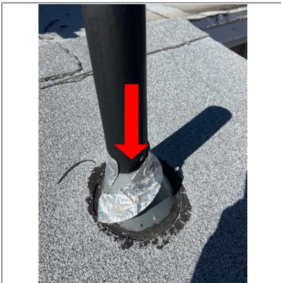
ITEM: 4:6. The sealant that was used around the back plumbing stack or vent at the roof is coming loose
