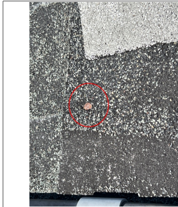
ITEM: 4:2. There are exposed and loose nails at the roofing material at one or more areas
