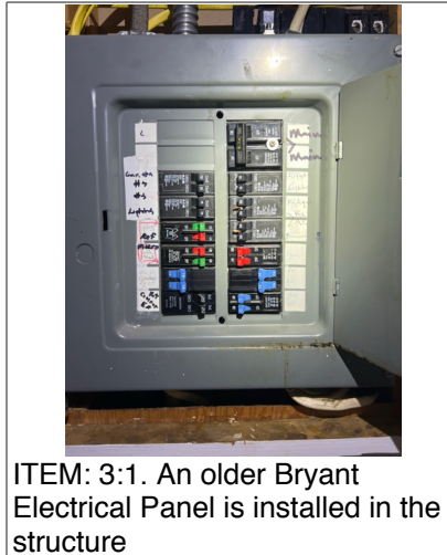
Image of electrical subpanel #3
