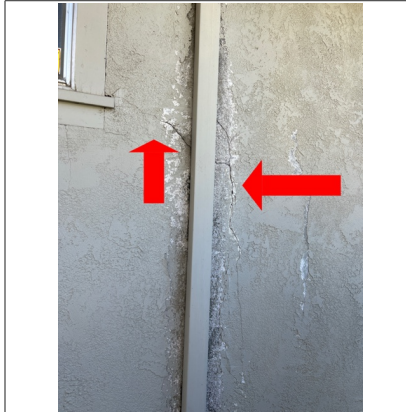
ITEM: 2:8. There are cracks noted in the stucco at various locations
