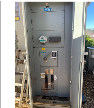
Image of the electrical service panel
