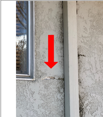
ITEM: 2:8. There are cracks noted in the stucco at various locations
