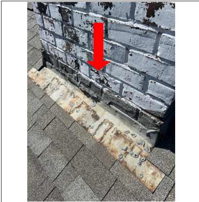
ITEM: 4:4. A section of the counter flashing at the chimney is missing
