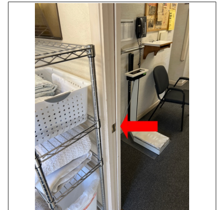
ITEM: 6:3. The pocket door at the back right hallway to kitchen area is stuck
