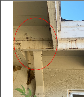
ITEM: 4:3. There is debris present on the roofing at the backside of the structure which appears to be obstructing the flow of water
