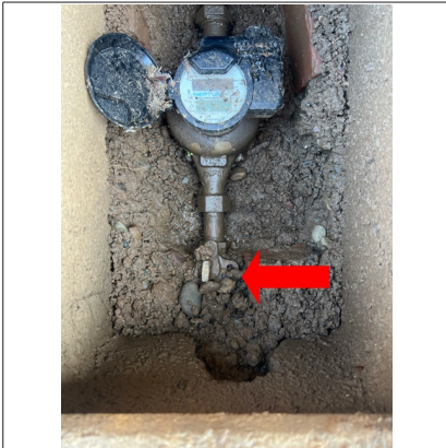
Image of the main water shut off valve in the service entry box
