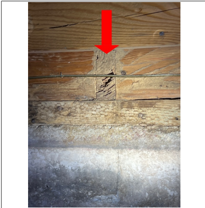
ITEM: 14:2. There is evidence of a wood pest infestation at the rim and floor joists
