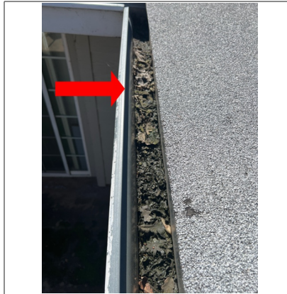
ITEM: 2:3. Portions of the insides of the gutters are full of debris and grass
