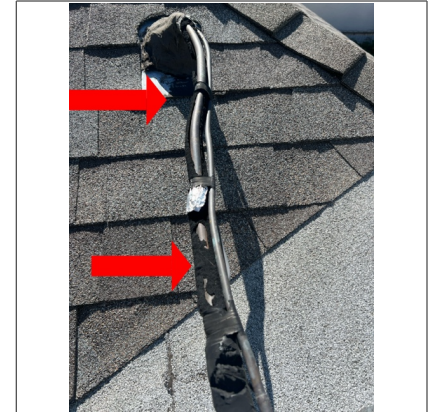
ITEM: 12:4. Sections of the insulation at the line set at both of the AC condensing units are torn and damaged
