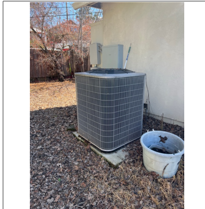
Image of AC condensing unit #2
