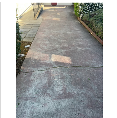
There are typical cracks present in the driveway
