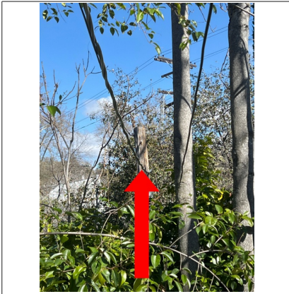
ITEM: 2:12. The electrical service entry wires are lower than 12 feet from the ground and are slightly in contact with some tree limbs
