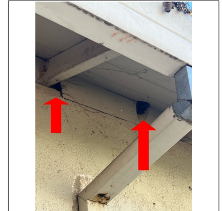
ITEM: 2:6. There are holes in the eaves at the back left corner of the structure
