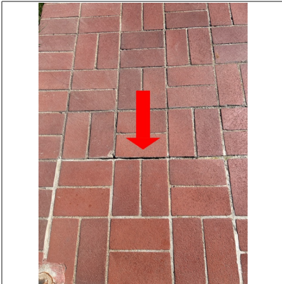
ITEM: 1:1. There is mortar missing at a small section of the front walkway
