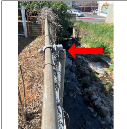
ITEM: 1:2. As with any fence that is built directly in the ground, there are damaged, worn, weathered and loose wood members present at various areas
