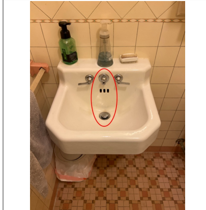
ITEM: 9:2. The stoppers at the back left and private bathroom sinks are not operable
