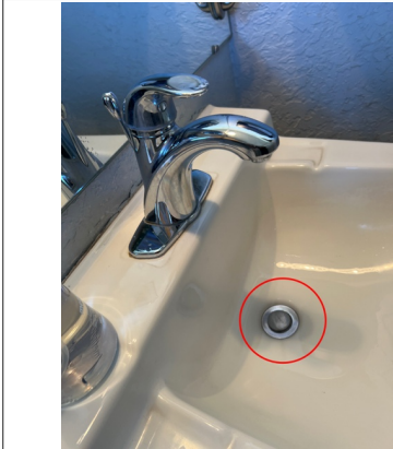
ITEM: 9:2. The stoppers at the back left and private bathroom sinks are not operable
