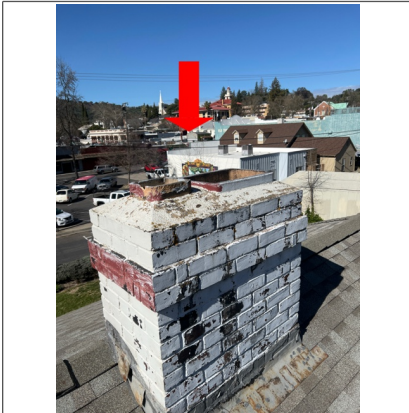
ITEM: 2:1. There was no rain cap installed at the top the chimney
