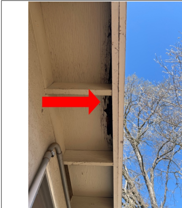
ITEM: 2:5. There is dry rot damage present at the back roof sheathing
