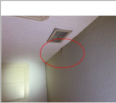
ITEM: 6:4. There are damaged and cracked sections of drywall throughout the structure
