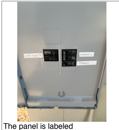
Image of electrical subpanel #2
