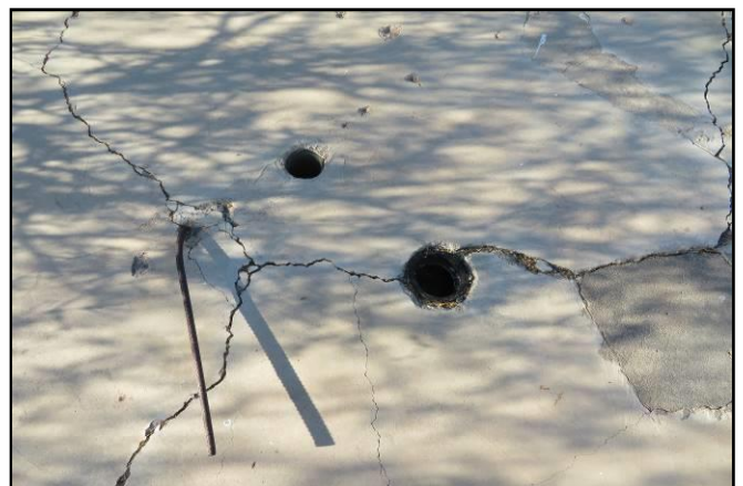
Picture 6 - One of the plumbing/utility pipes on one of the larger concrete slabs on the southeast portion of the Property.
