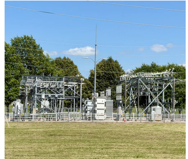
Ameren substation on east side of the property
