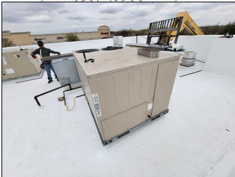
18 : Representative HVAC unit.
