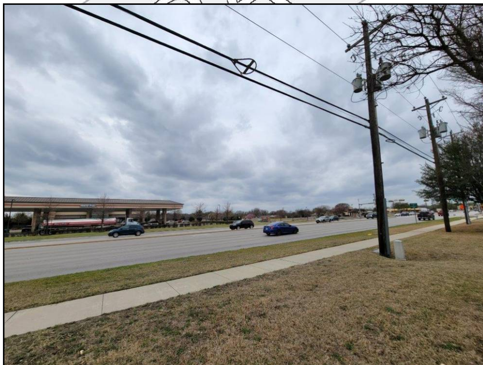
24 : Off-site pole-mounted transformers.
