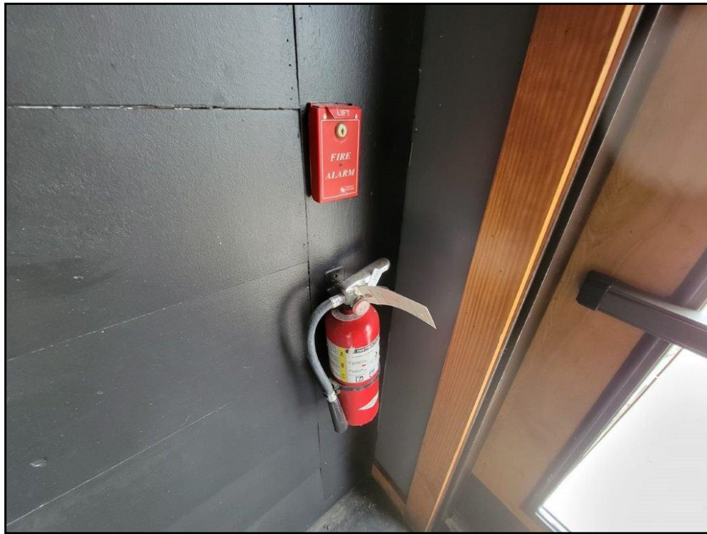
29 : Pull station and fire extinguisher.
