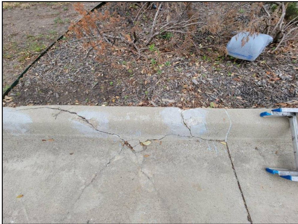
9 : Damaged curbing at southeastern corner of site.
