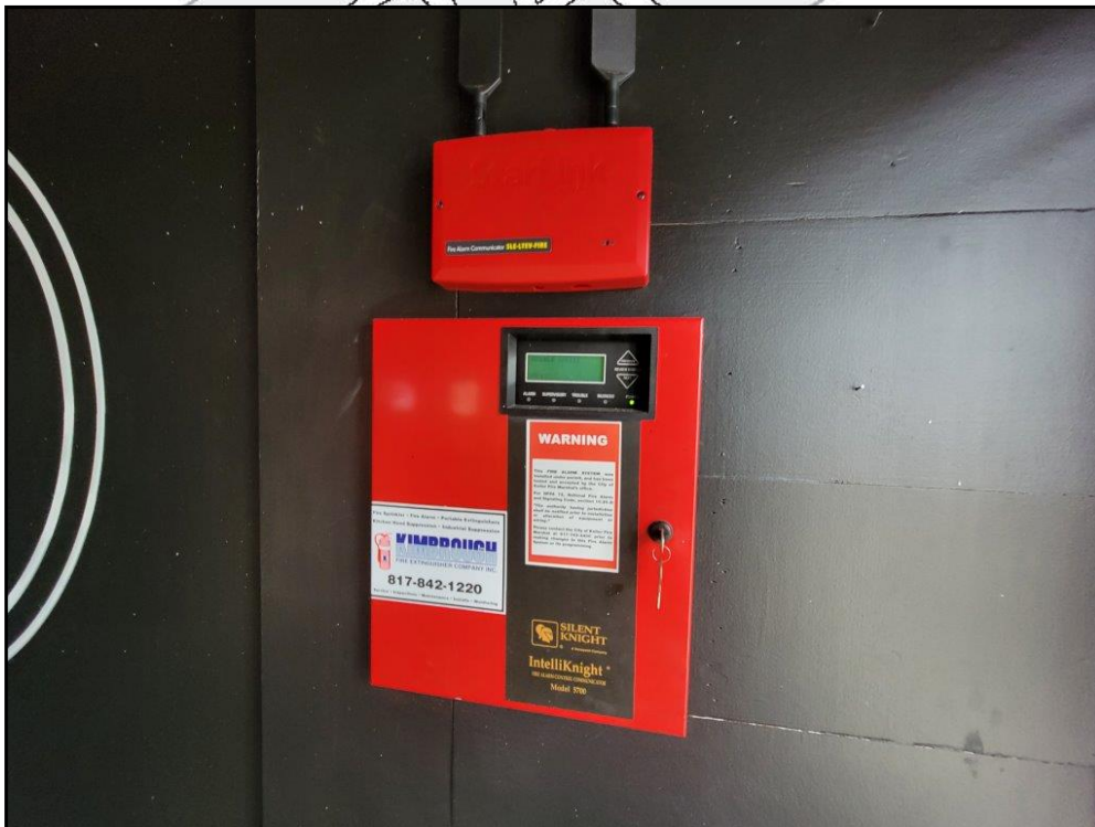
28 : Fire alarm control panel.
