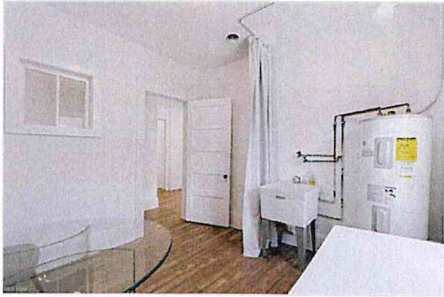
Utility room featuring water heater
