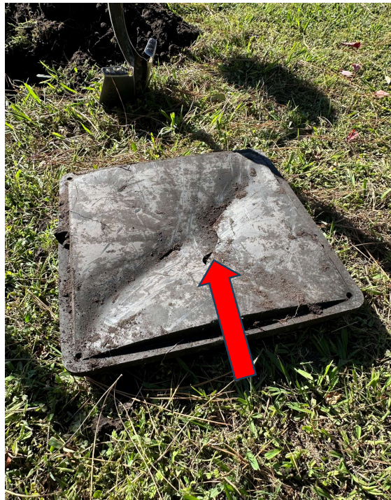
Distribution box lid
