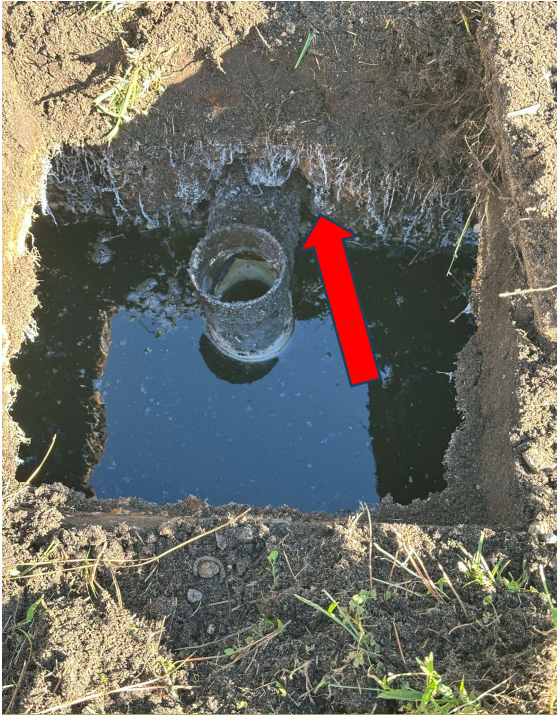
Septic tank outlet
