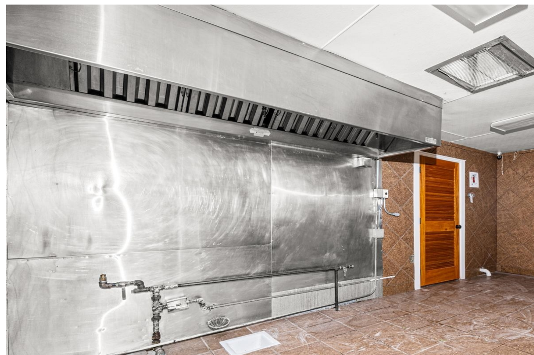
Hood Vent in Place
