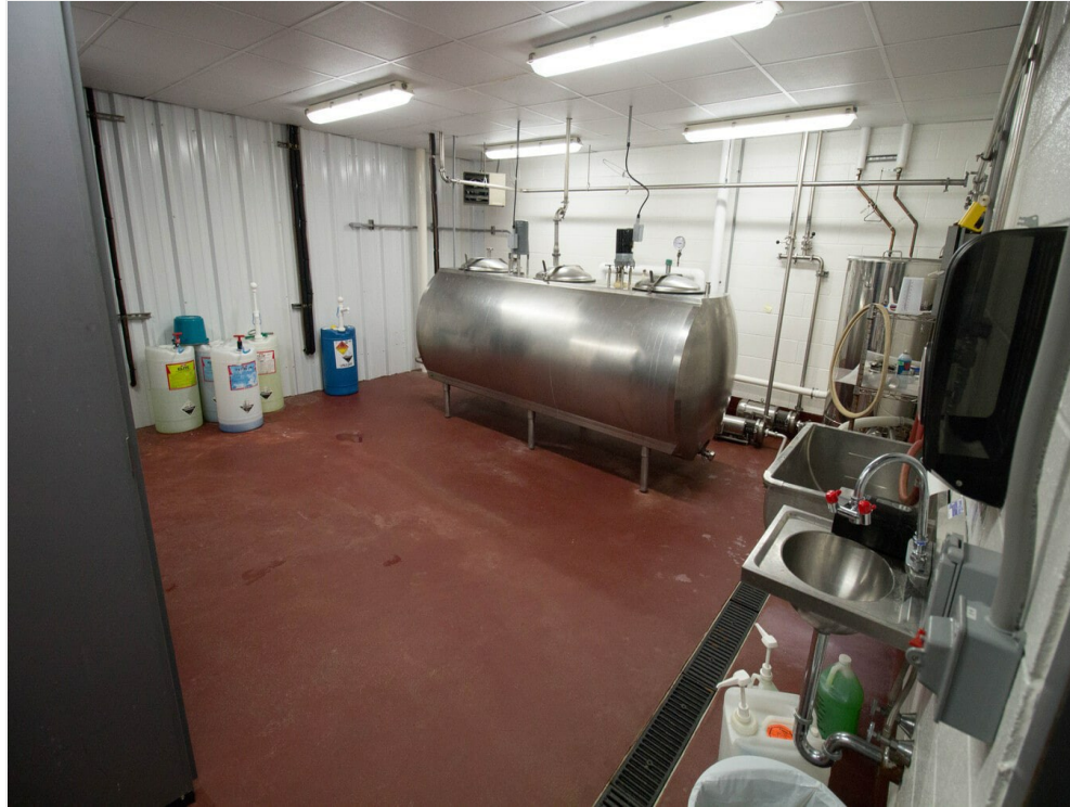
Raw milk processing room with CIP system
