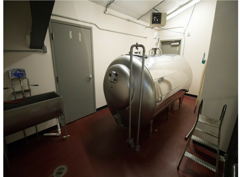
Second story bulk tank
