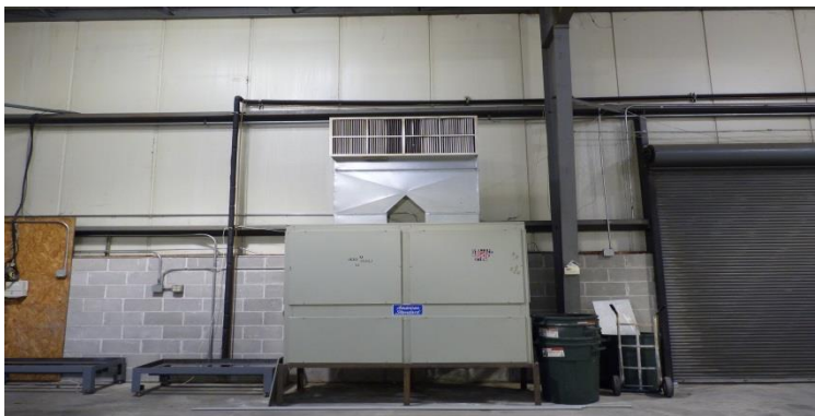
TRANE A/C SYSTEM COOLS WAREHOUSE
